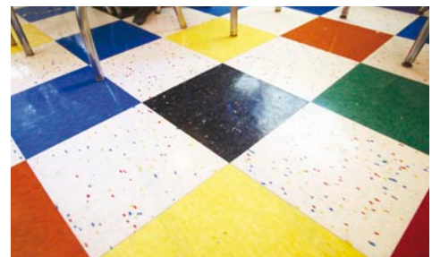
Asbestos-containing floor tiles
